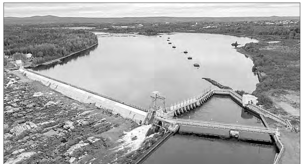
Rehabilitation of the main dam at Grand Falls for Newfoundland and Labrador Hydro is complete.
