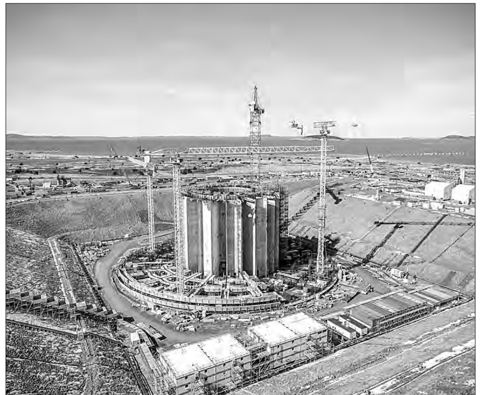
The West White Rose Project recently reached an important milestone with the completion of the base slab of the gravity-based structure.
