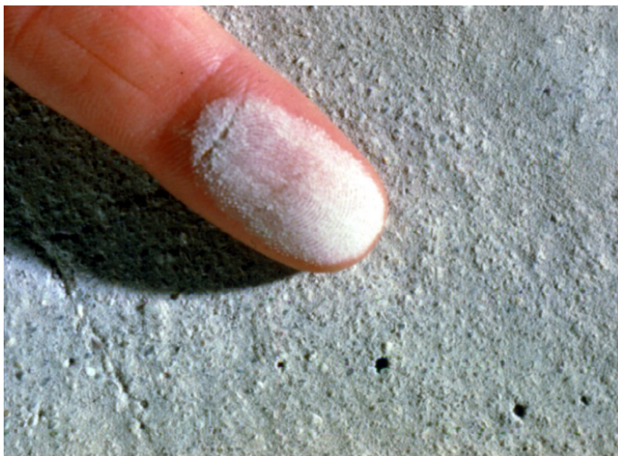
Dusting on Concrete Surface
