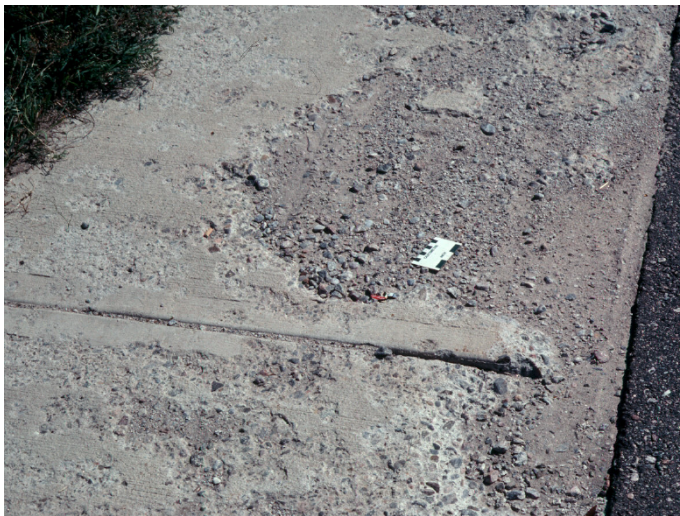
Scaled Concrete Sidewalk
