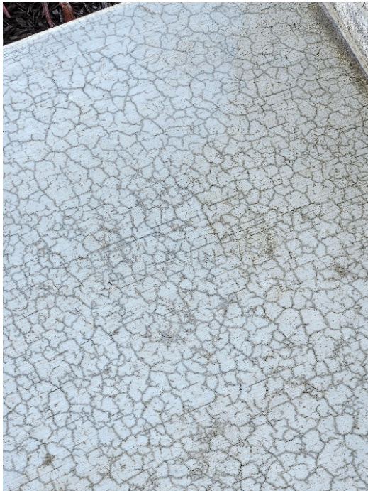
Example of concrete crazing
