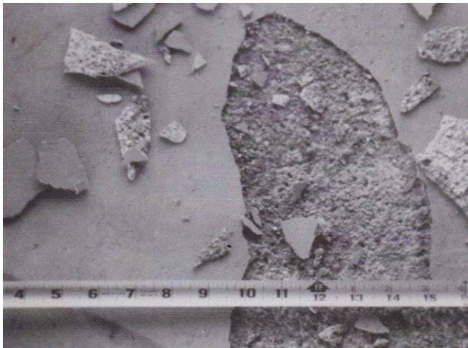
Example of Delaminated Concrete
